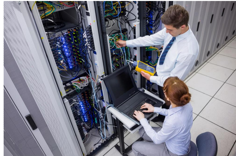
Nord-Micro Datacenter local side Germany/Frankfurt
