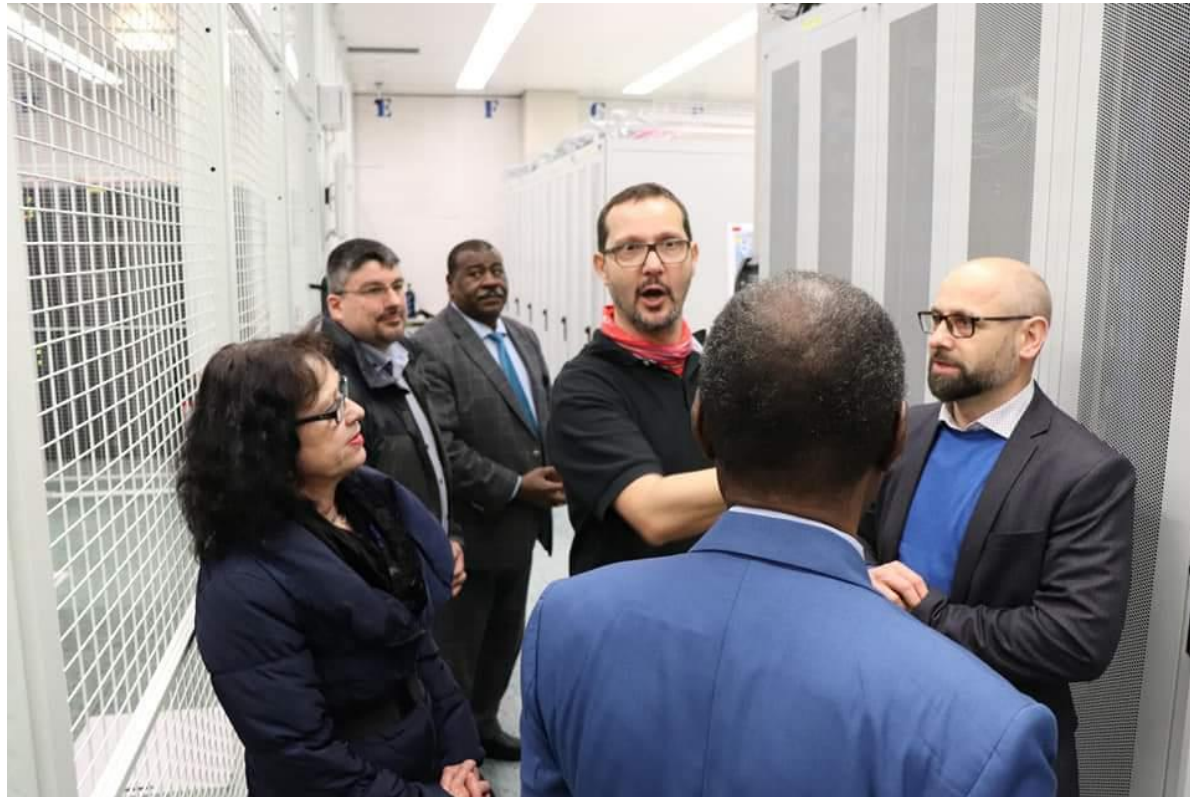
GGSC Partner Diamond in UZH Datacenter
