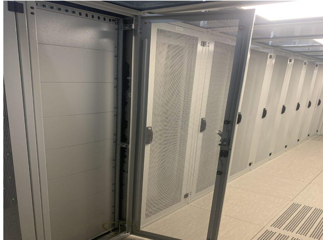
Datacenter Trusted Colo
