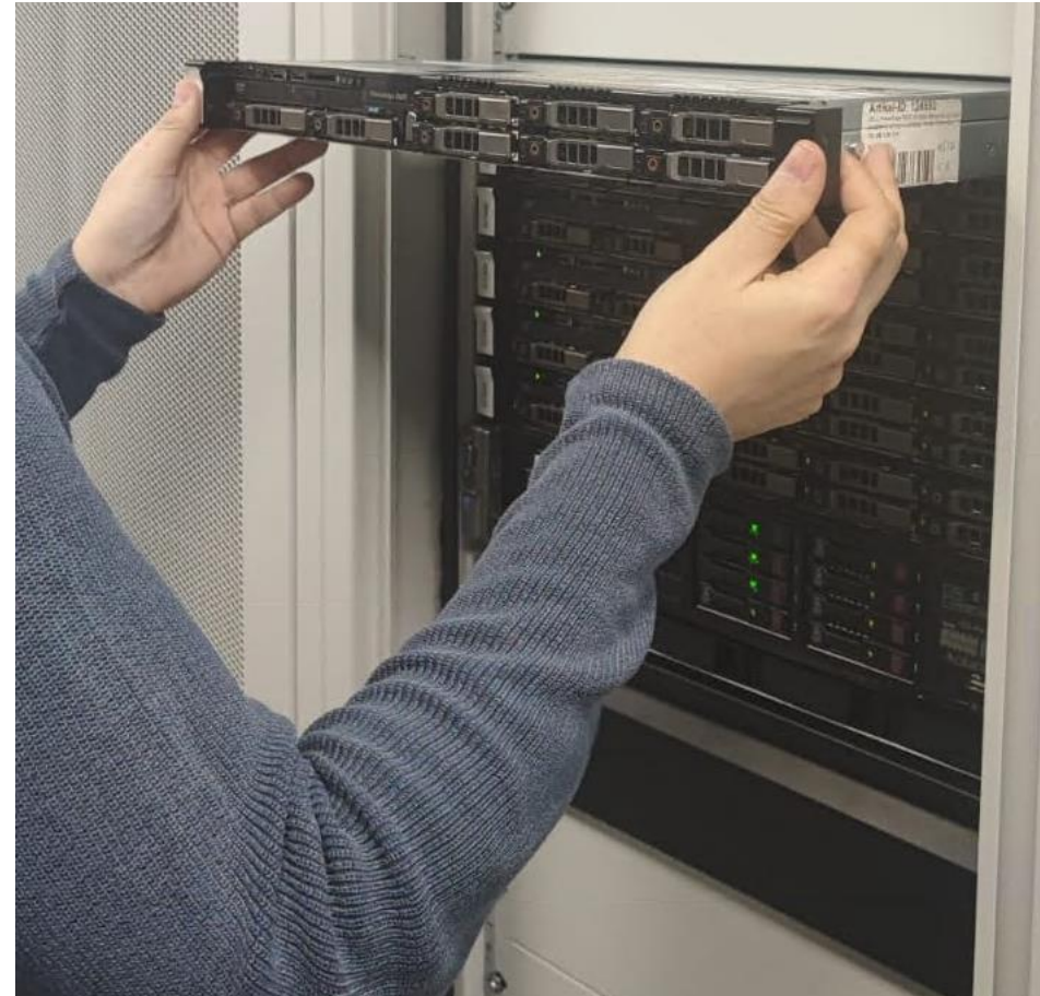
Datacenter Trusted Colo
