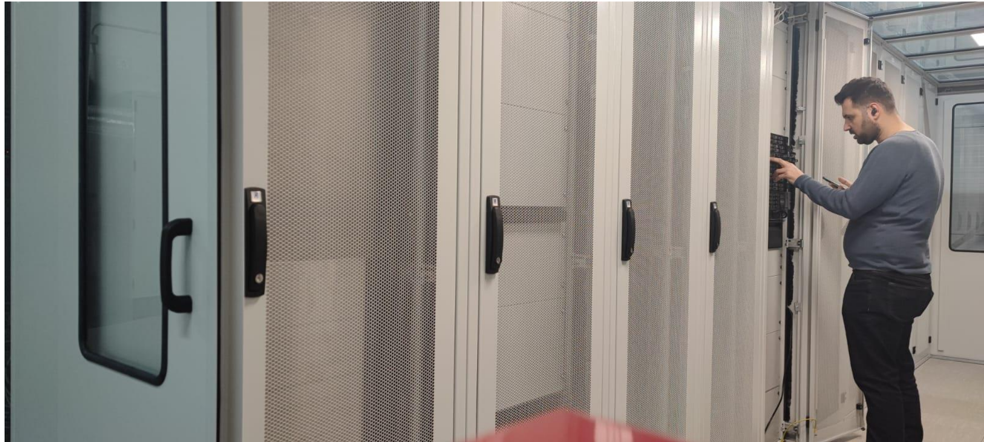
Datacenter Trusted Colo
