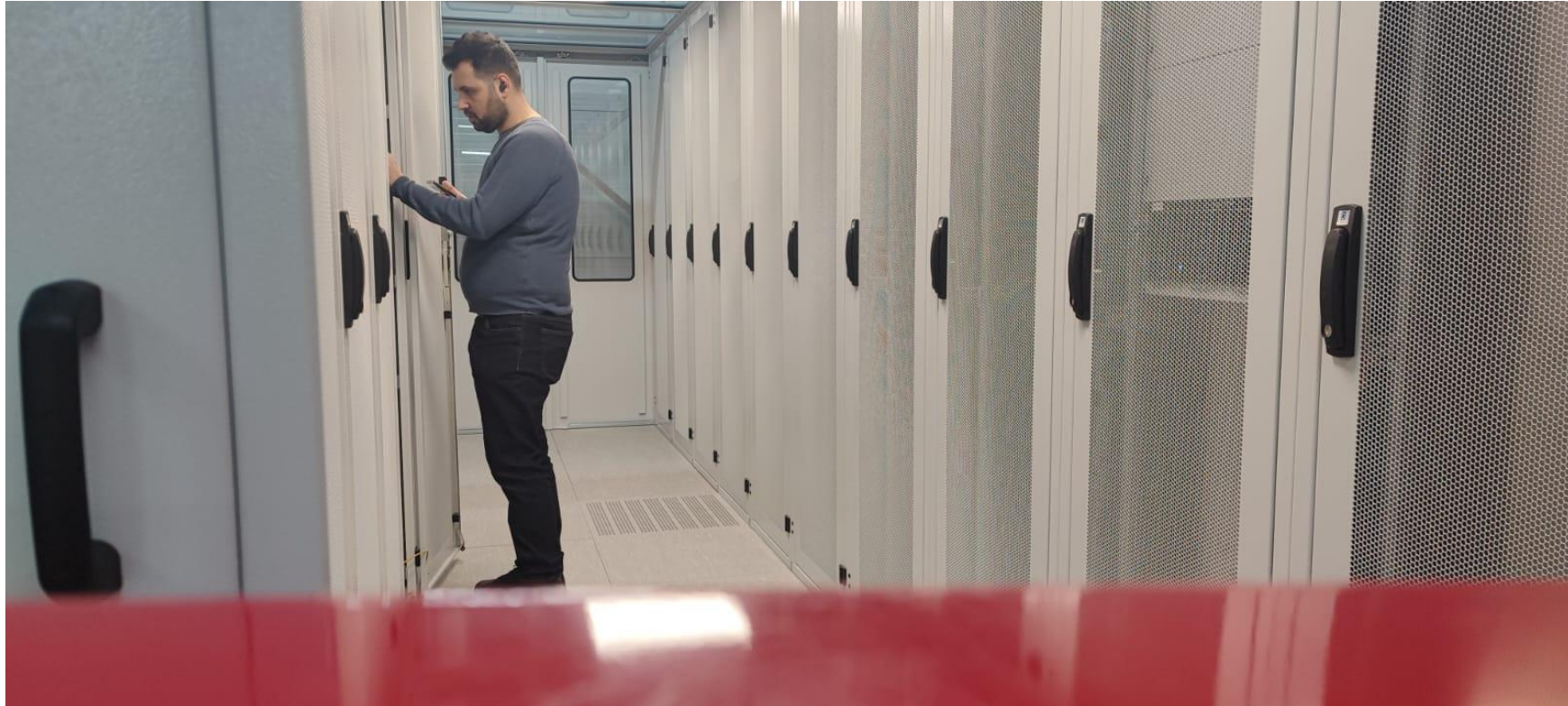
Datacenter Trusted Colo
