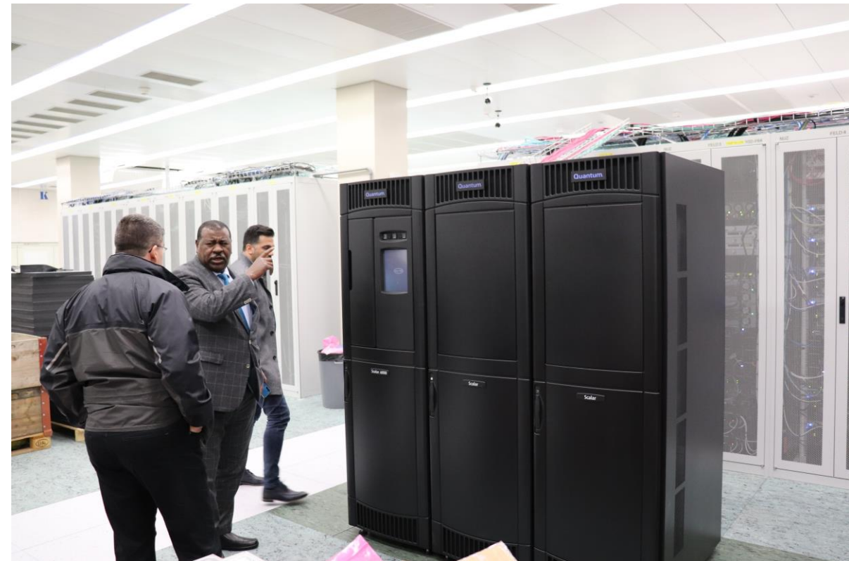
GGSC Partner Diamond in UZH Datacenter
