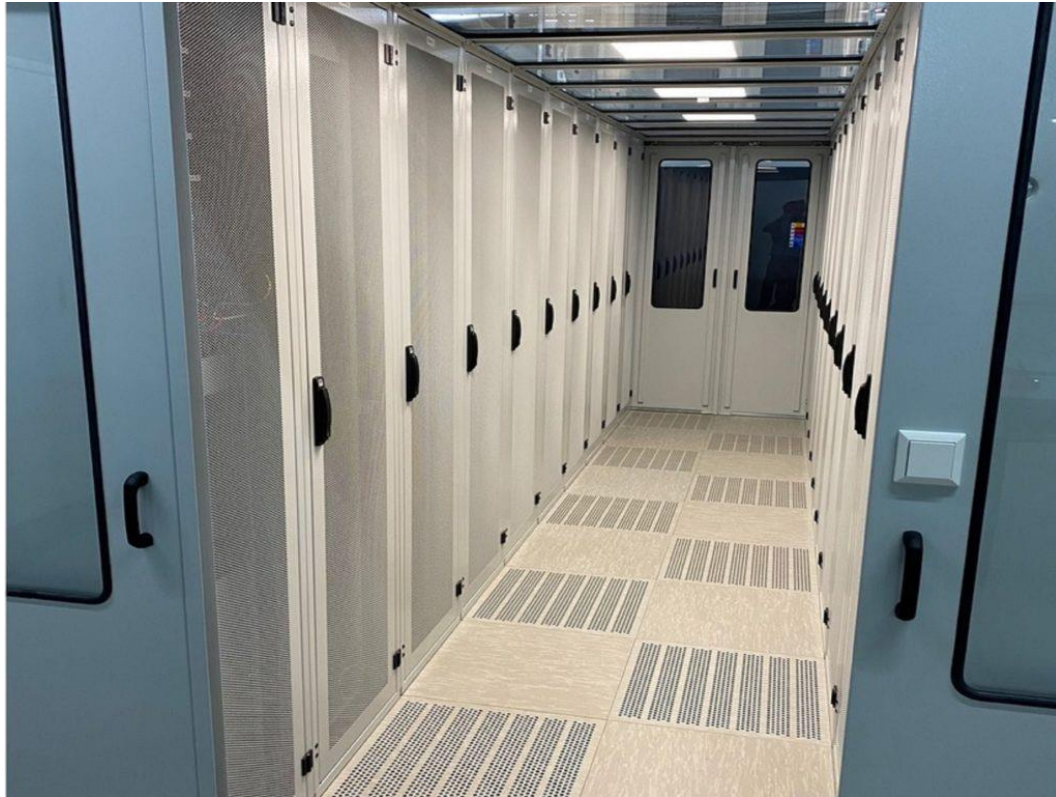
Datacenter Trusted Colo
