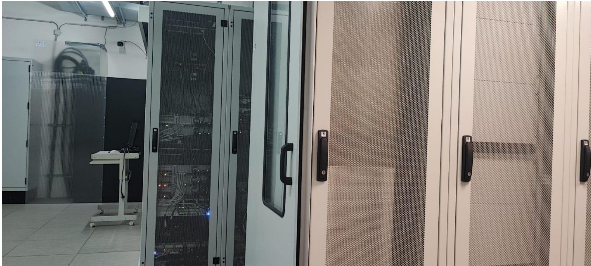
Datacenter Trusted Colo
