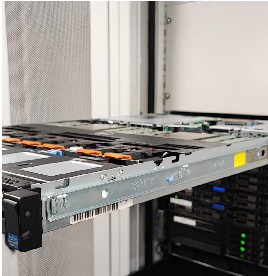
Datacenter Trusted Colo
