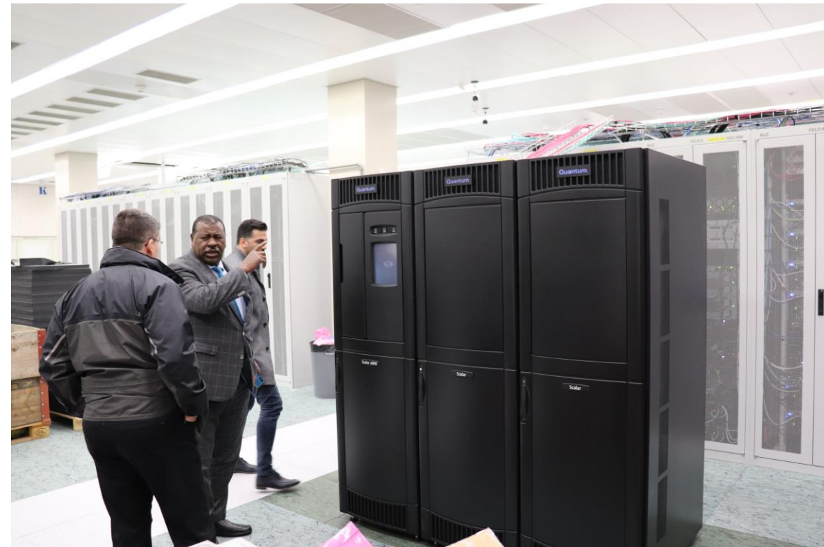
GGSC Partner Diamond in UZH Datacenter
