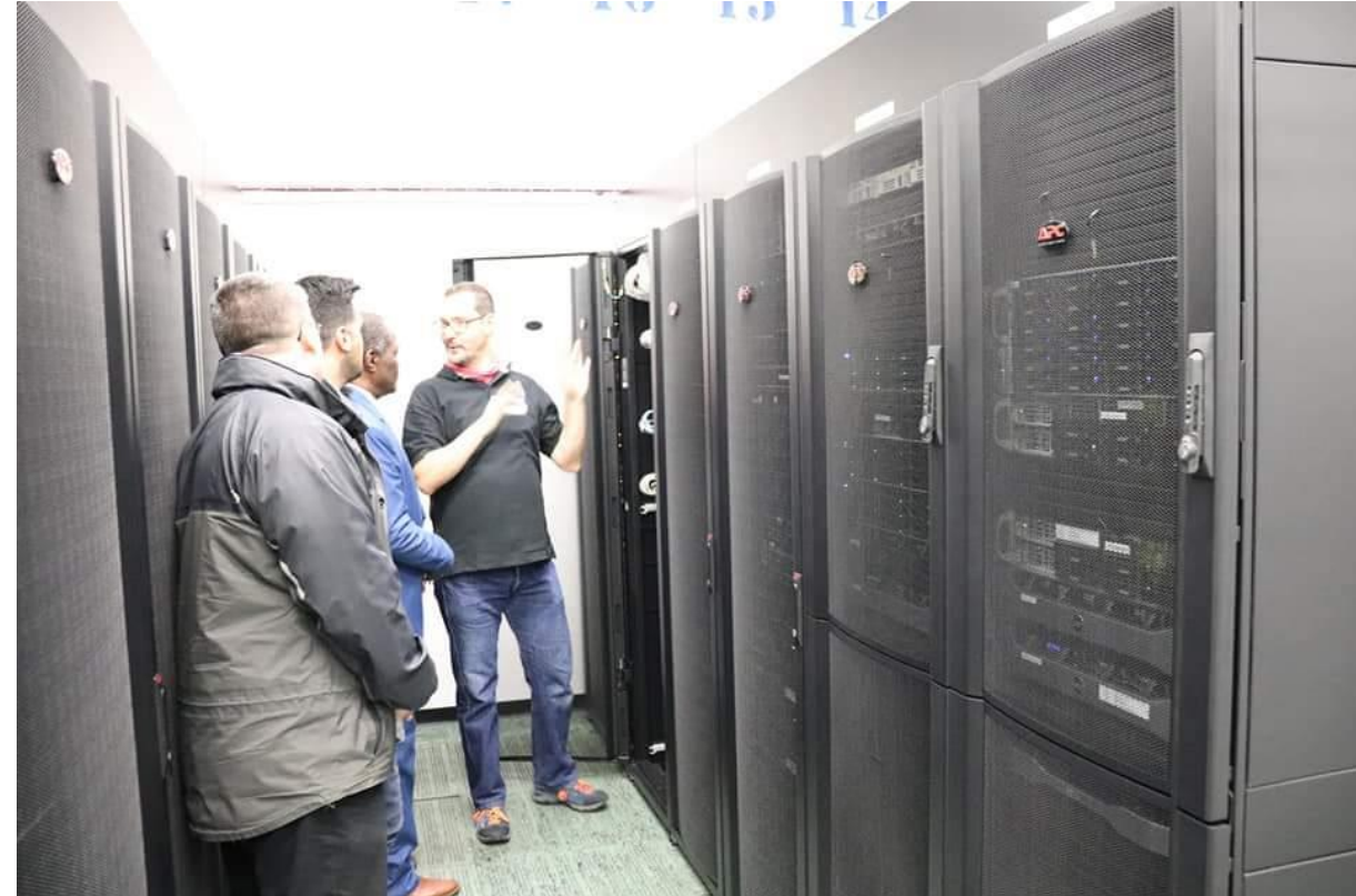
GGSC Partner Diamond in UZH Datacenter
