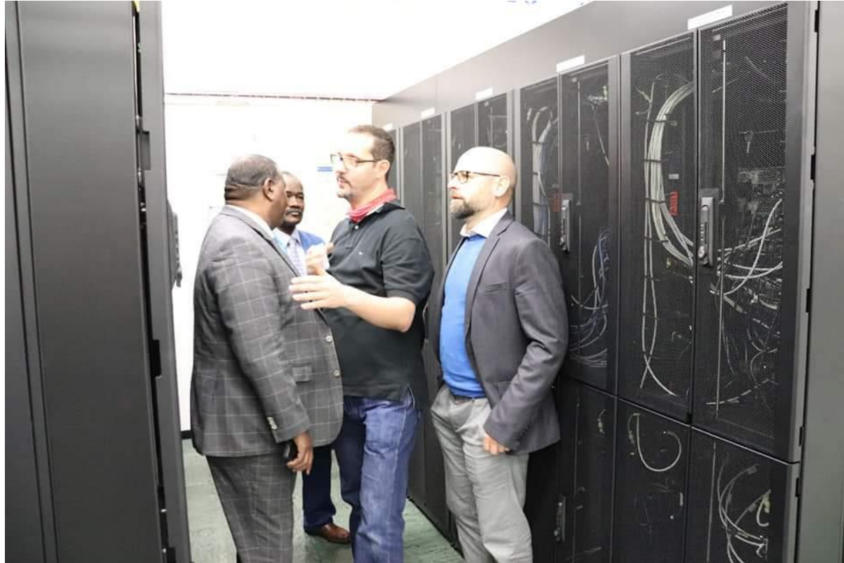
GGSC Partner Diamond in UZH Datacenter
