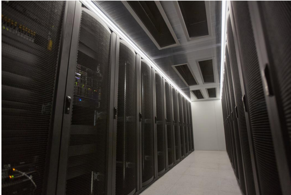
Clariant Innovation Center Datacenter local side Germany/Frankfurt
