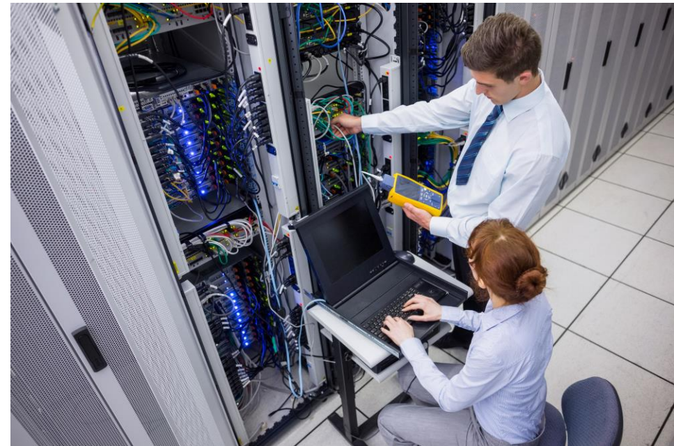
Nord-Micro Datacenter local side Germany/Frankfurt
