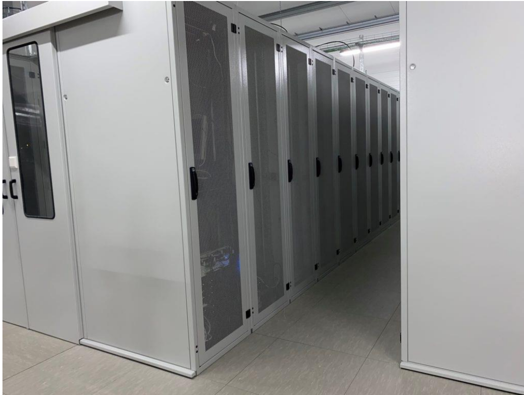
Datacenter Trusted Colo
