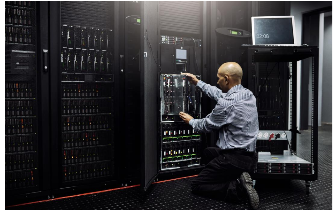
Datacenter side UBS Bank in Germany/Frankfurt
