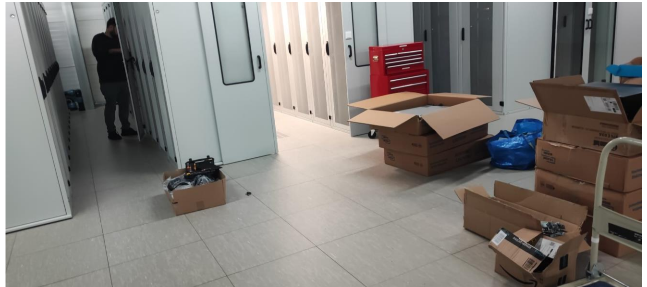
Datacenter Upgrade with high Performance Servers
