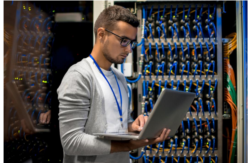
Clariant Innovation Center Datacenter local side Germany/Frankfurt
