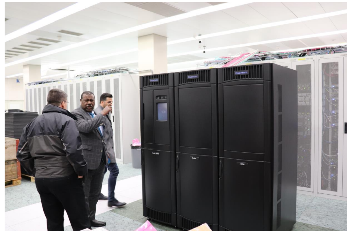
GGSC Partner Diamond in UZH Datacenter
