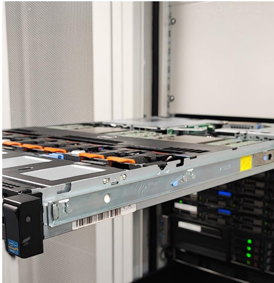
Datacenter Trusted Colo
