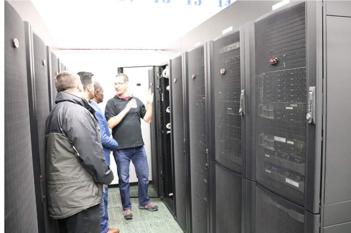
GGSC Partner Diamond in UZH Datacenter
