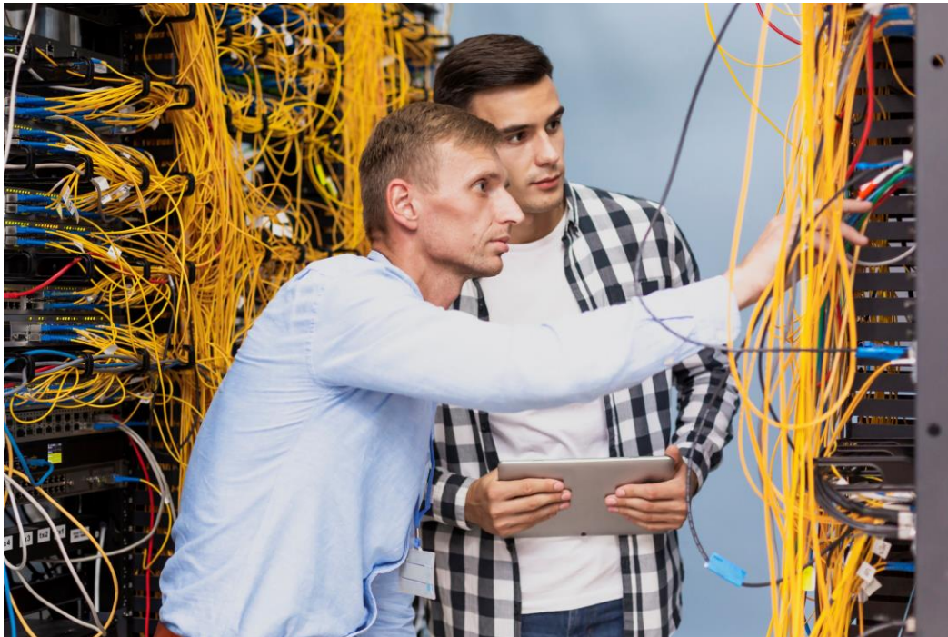
Datacenter local side UBS Bank in Germany/Frankfurt
