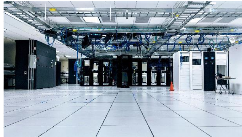
Data Center Interior
