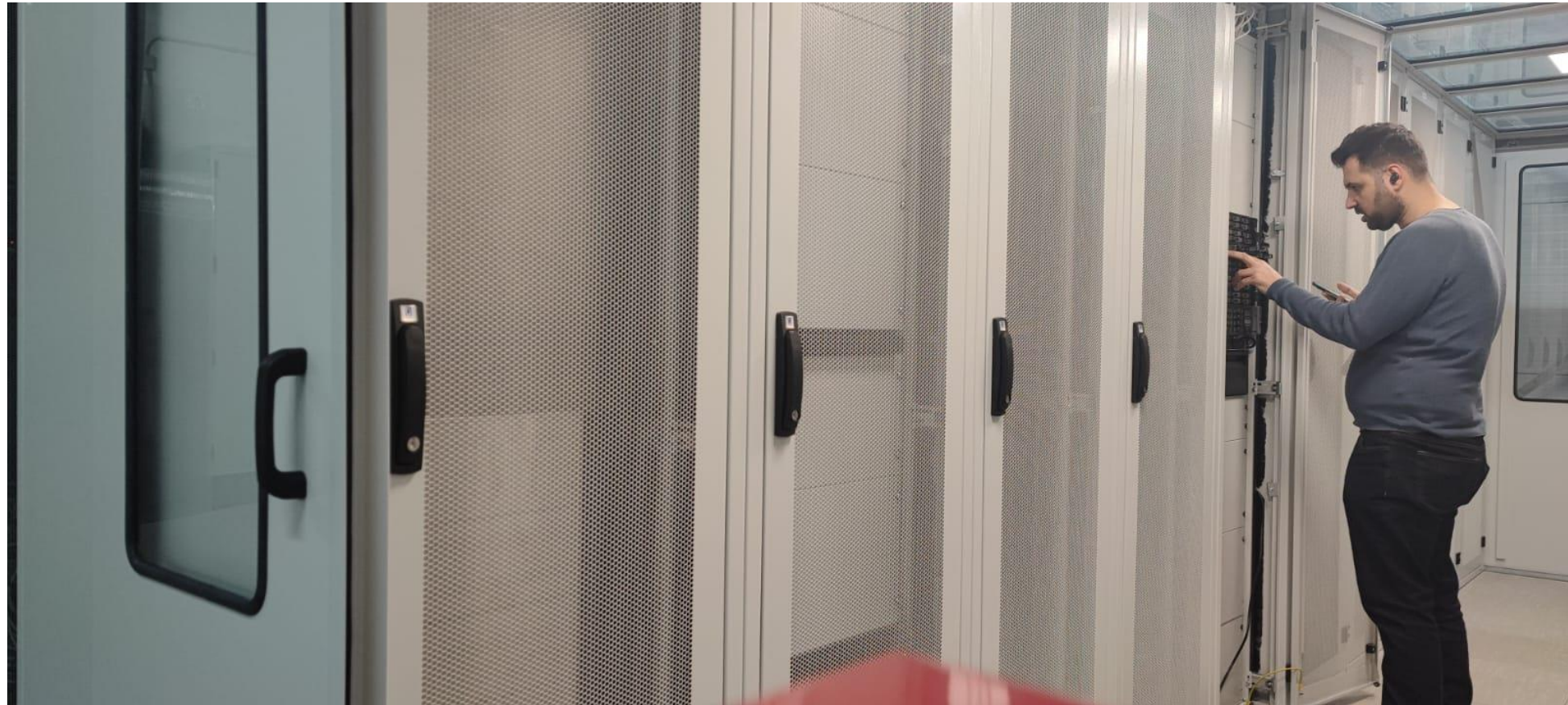
Datacenter Trusted Colo
