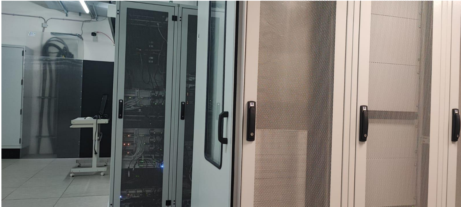
Datacenter Trusted Colo
