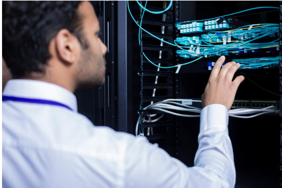
Nord-Micro Datacenter local side Germany/Frankfurt
