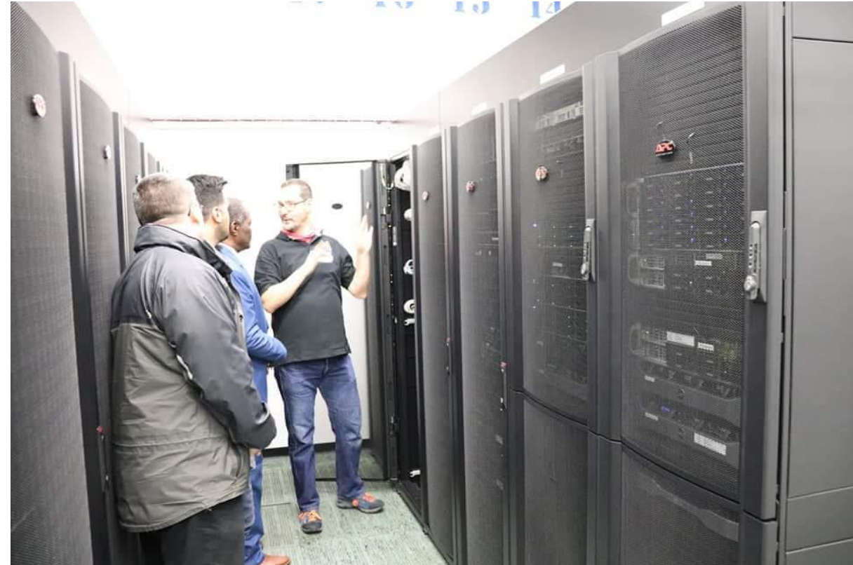
GGSC Partner Diamond in UZH Datacenter
