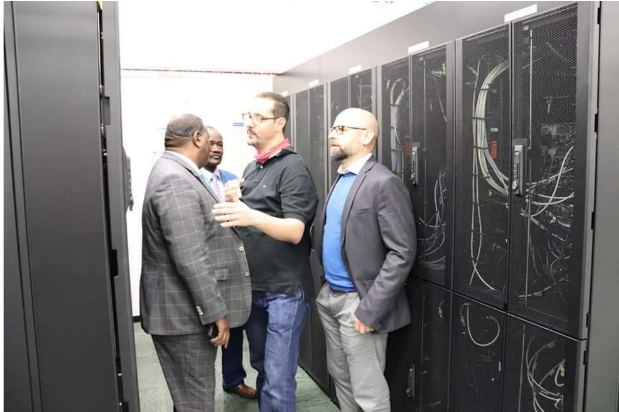
GGSC Partner Diamond in UZH Datacenter
