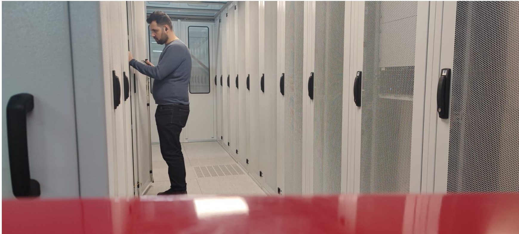
Datacenter Trusted Colo
