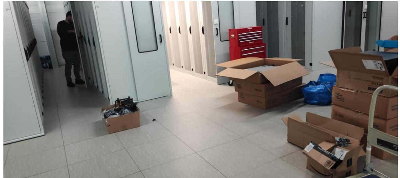
Datacenter Upgrade with high Performance Servers
