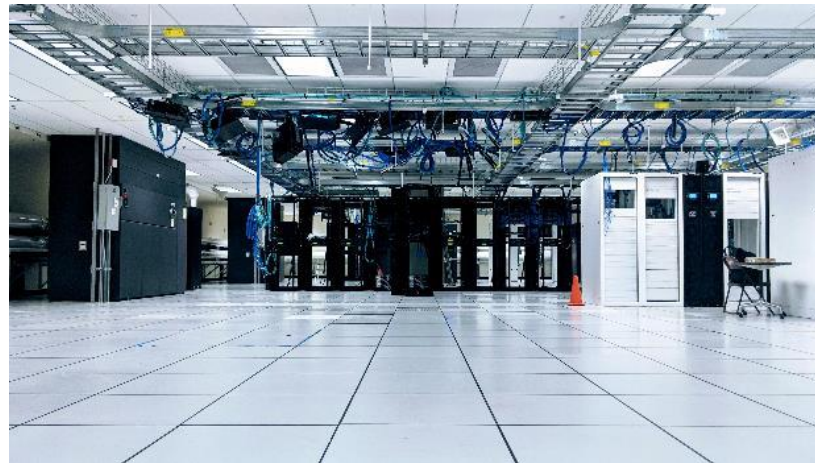
Data Center Interior
