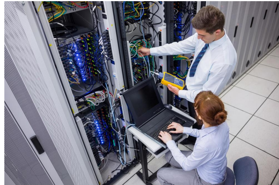
Nord-Micro Datacenter local side Germany/Frankfurt
