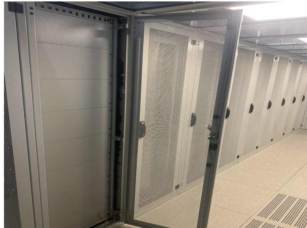
Datacenter Trusted Colo
