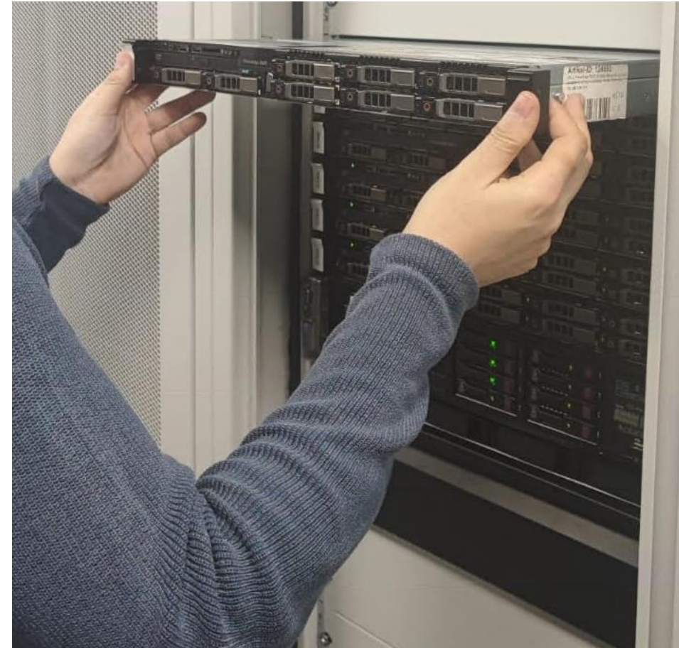
Datacenter Trusted Colo
