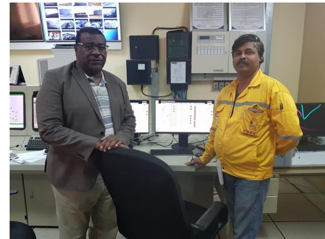
SCADA used for Process Control
