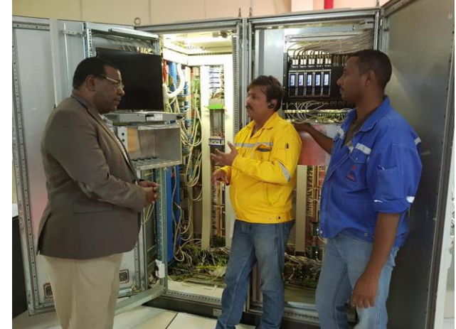
Plant Control System Infrastructure
