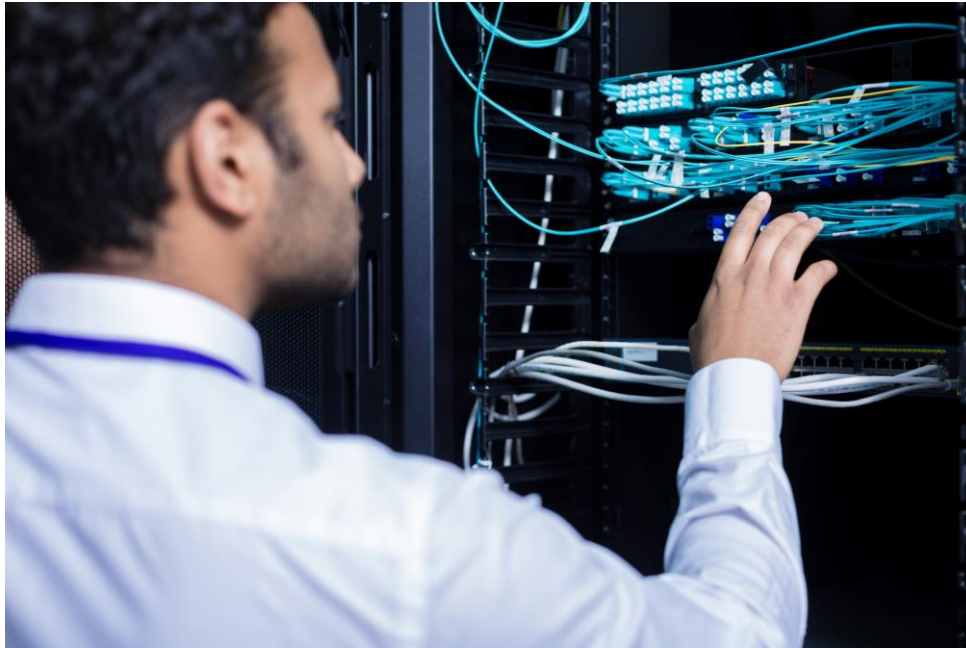
Nord-Micro Datacenter local side Germany/Frankfurt
